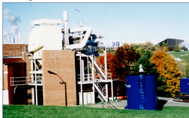
Demonstration Boiler Site with Baghouse, Ceramic Filter, and Duct Sorbent Injection Systems
